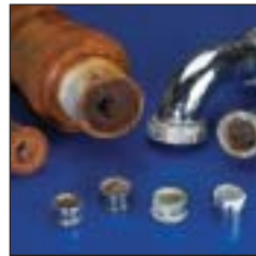
Scale buildup can become a costly problem over time
